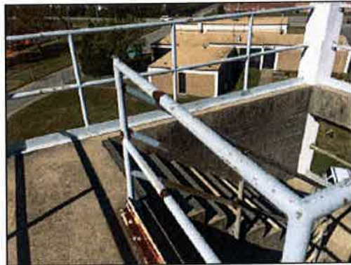
Photo 7 Worn/Damaged Hand Rail
