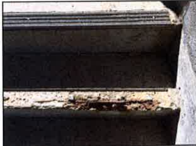
Photo 3 Exposed Tread Nosing Bar
