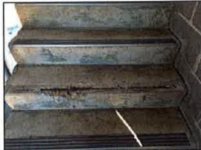
Photo 4 Exposed Tread Nosing Bar
