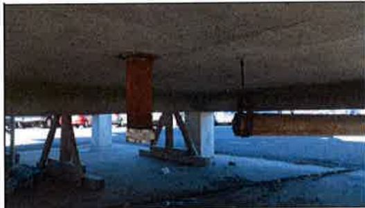
Photo 1 Sanitary Piping Missing
