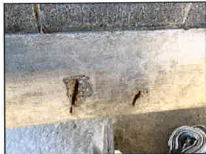
Photo 2 Typical Concrete Spall
