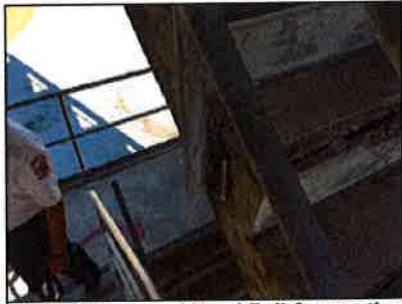
Photo 6 Displaced Hand Rail Connection
