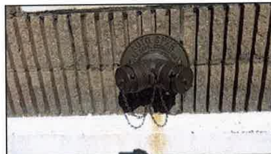
Photo 6 Existing Hose Connection
