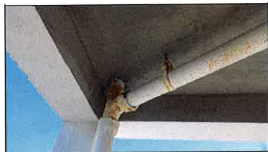
Photo 3 Deteriorated Sanitary Piping
